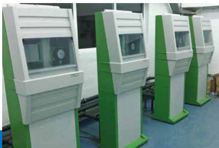
Chlorine Gas Dosing Facility
