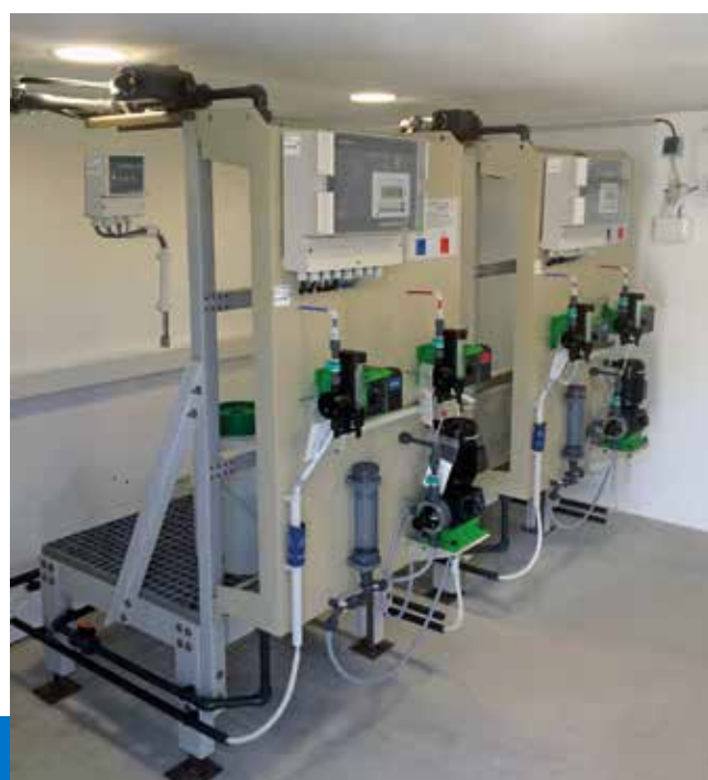
Chlorine Dioxide Generators
